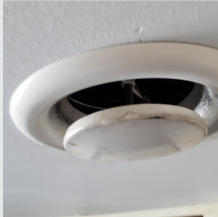
Bathroom ventilation air supply with air inlet adjustment
